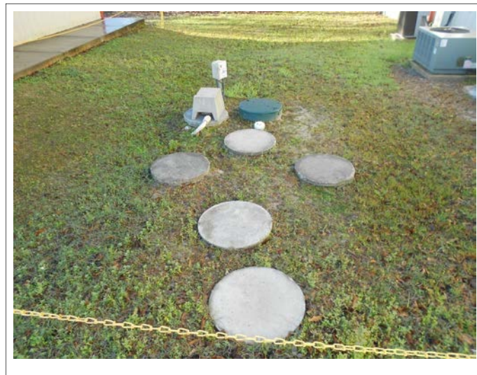
Portions of the septic system associated with the office building.
