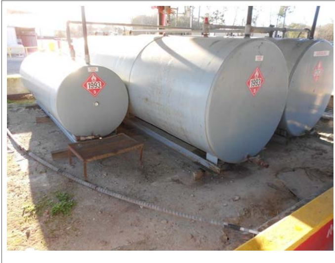
Three (3) AST located within fueling area.
