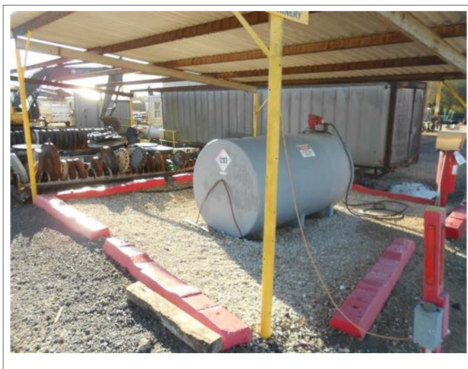
1,000-gallon off road diesel AST located on the western portion of the subject property.
