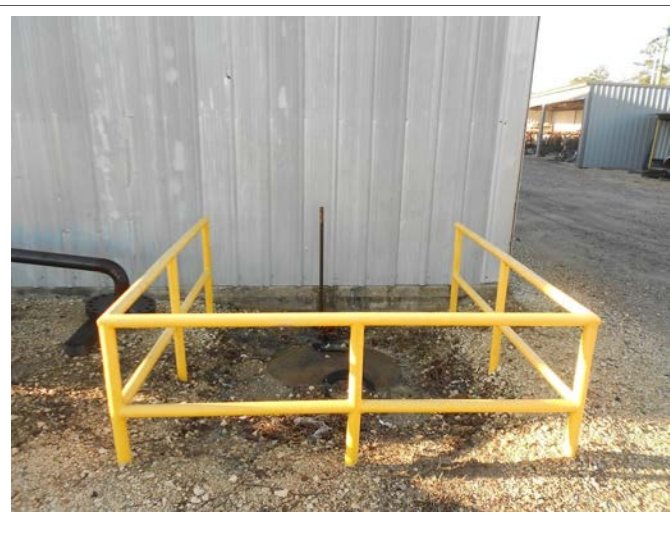
Portion of the septic system associated with the shop building.
