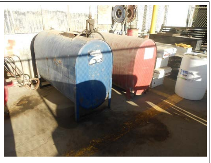
Used oil ASTs with staining located on the outside of the shop building.
