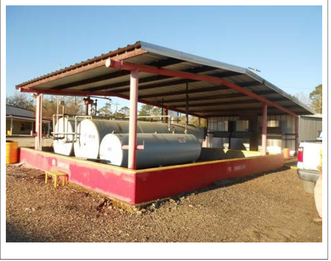
Fleet fueling area.
