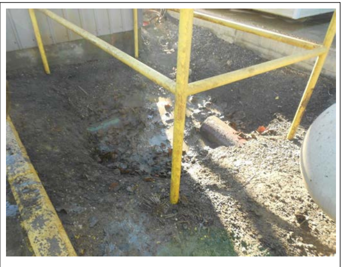
Earthen ditch in the central portion of the property near the eastern vehicle wash area.
